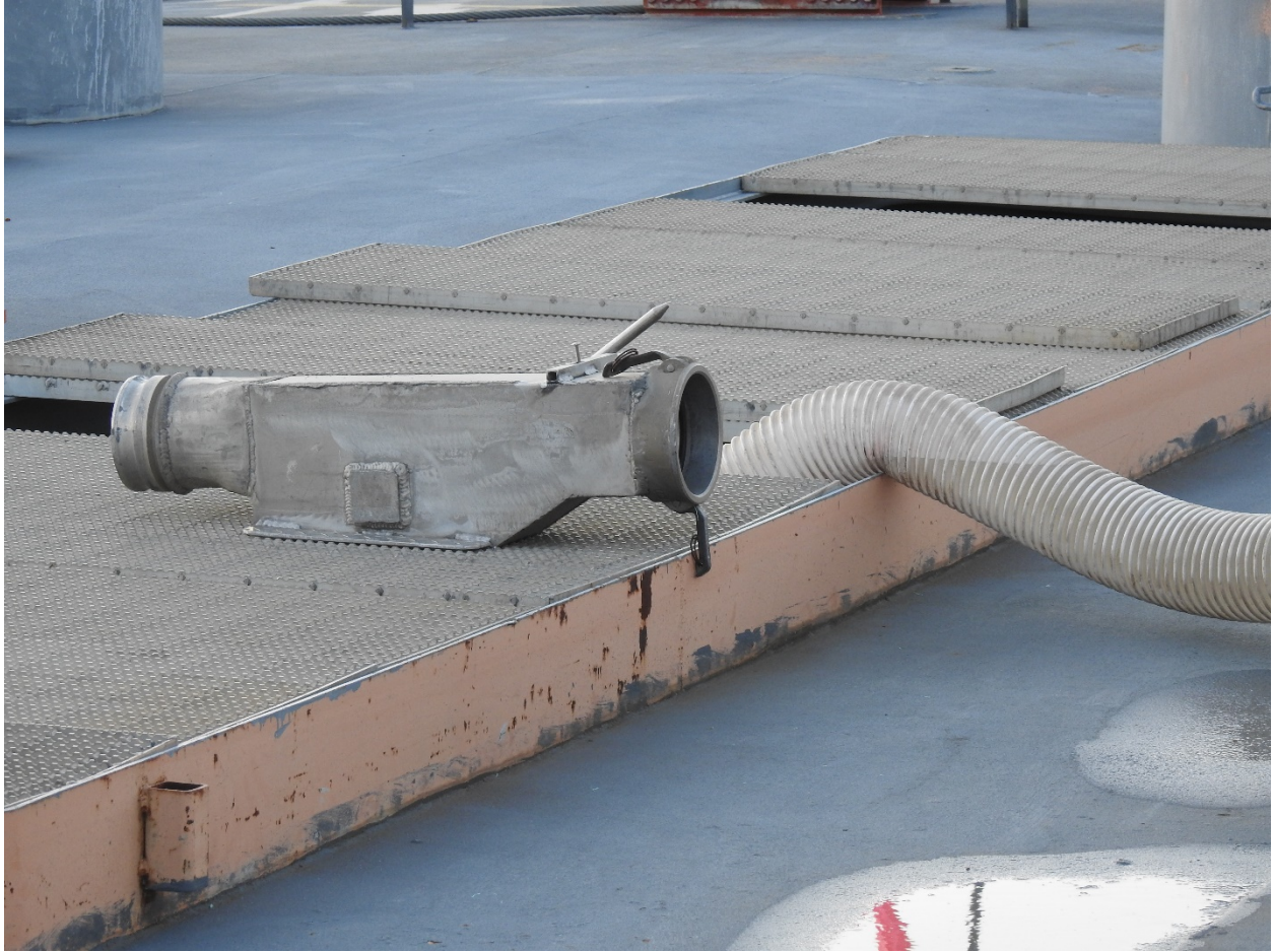
Image 1: Cam lock fitting mounted on transport barges.
